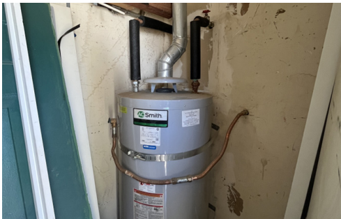
Thermostat (top) and Water Heater (bottom)
