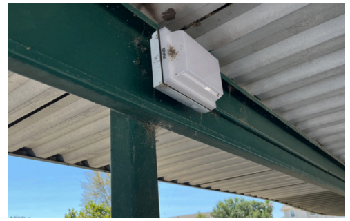
After: Parking LED Fixture
