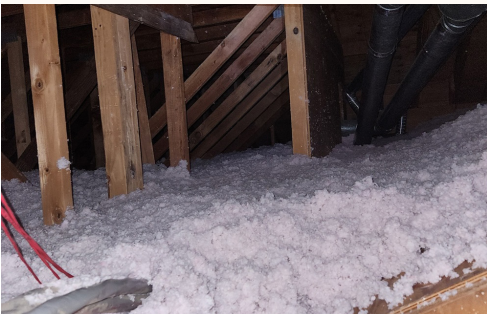
Ceiling Lighting (top) and Attic Insulation (bottom)
