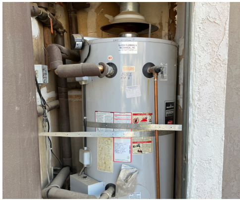
BEFORE: Gas Tank Water Heater
