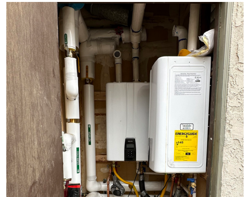
AFTER: Tankless Water Heater
