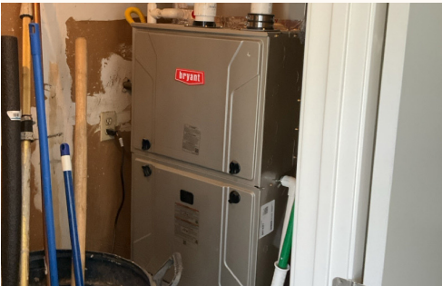
Thermostat (top) and HVAC Furnace (bottom)
