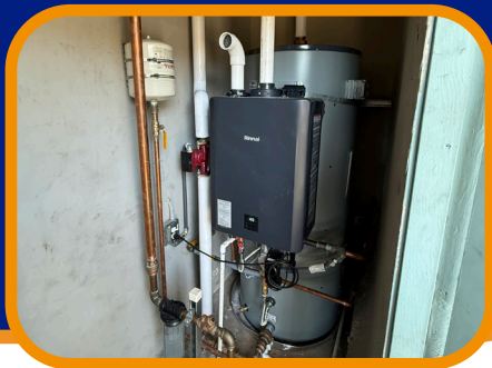
Tankless water heater, Pasadena, CA
