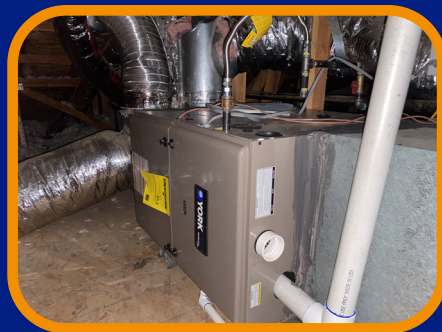
HVAC furnace, Sacramento, CA
