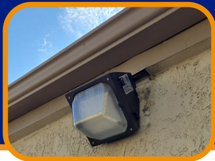
LED lighting upgrade, Baldwin Park, CA
